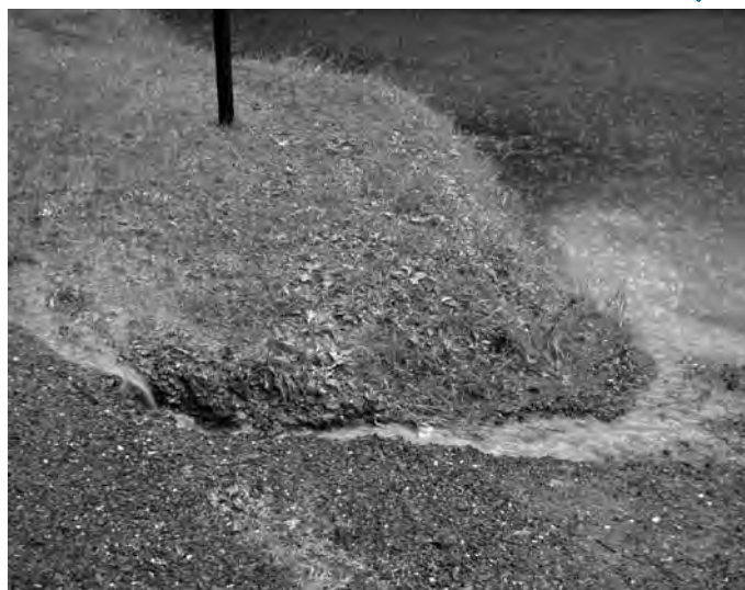
Erosion of poorly graded dirt and gravel roads such as this one in Barnet, Vt., can deliver sediment to streams after heavy rain.
